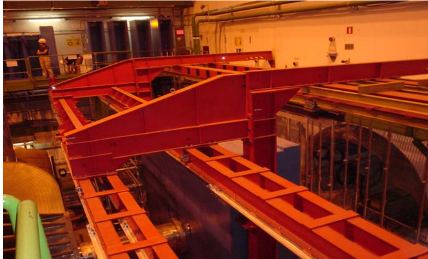
Fig. 9. Superstructure for support of the tracking and trigger chambers designed by the PNPI group
